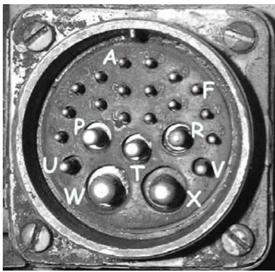
Socket on generator, significant pins. The AC outlet for power tools from pins P, R & T is rarely used. This is identical to the connector that plugs into Socket 1 on Generator Panel.
