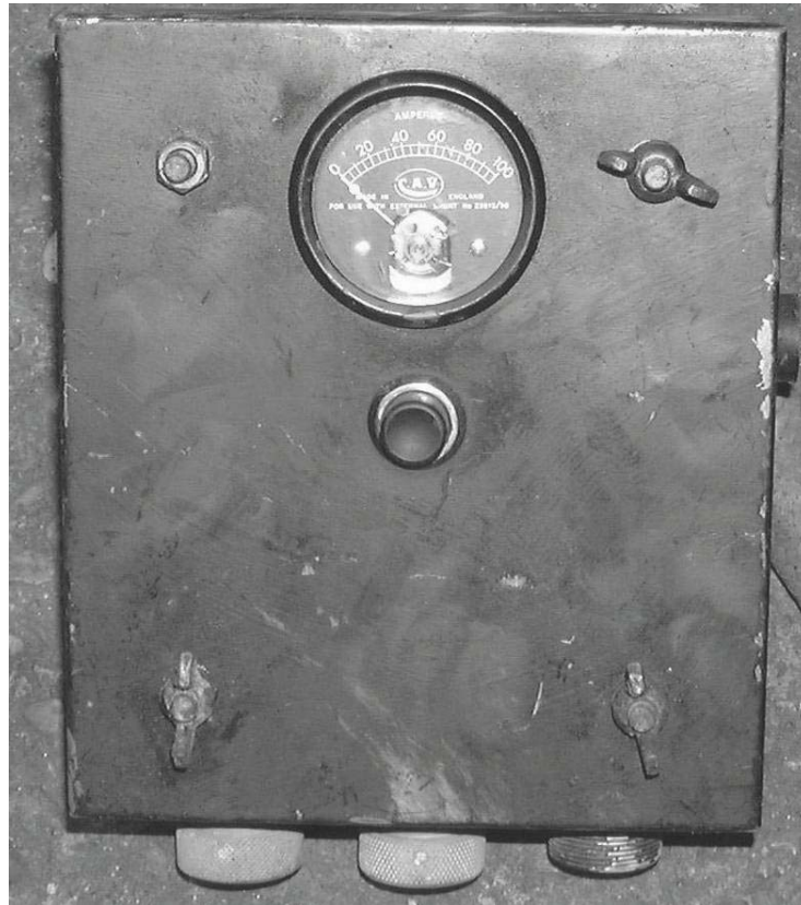
The shunt box for the transistorised regulator.
